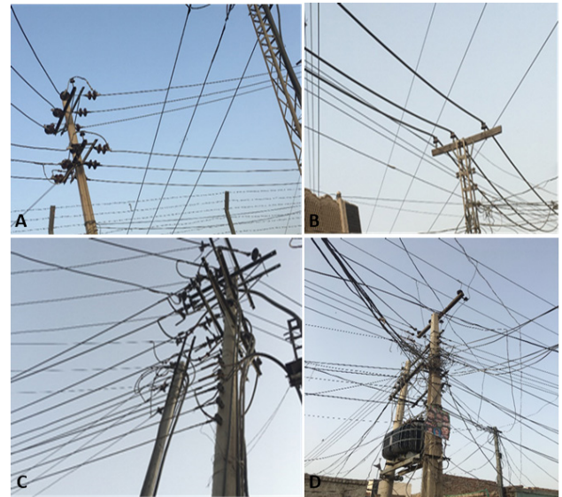
Fig. 3. Suspended wire on 11kV Tata Pur Feeder (A), 1000MCM cable is used in 11kV line (B), Dangerous Pole (11kV) (C) and Dangerous Pole (400V) (D).
